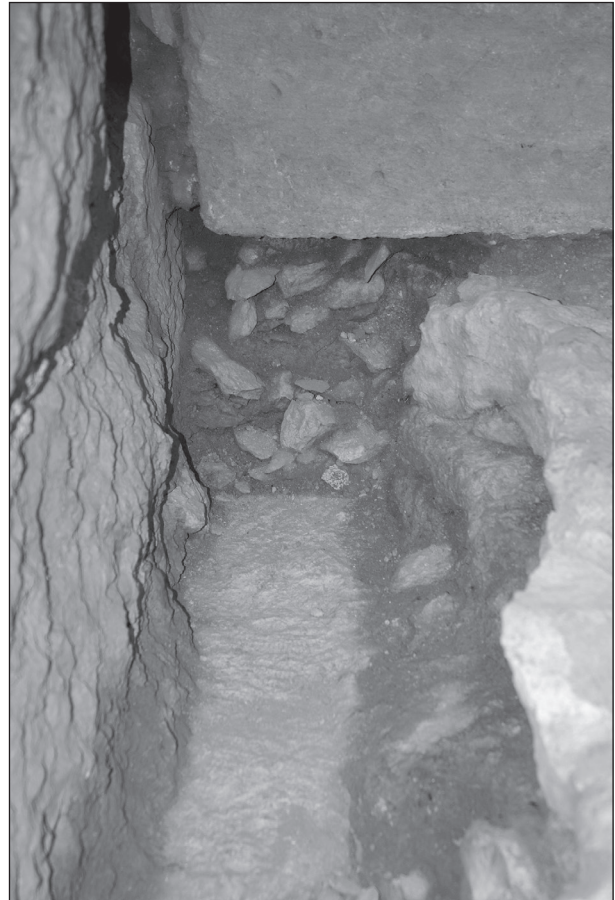
6. Southern vault under the pronaos. Detail of the foundation trench US18049 from north after the investigation of the fill, still visible in the section under the southern wall of the vault, covering the offset foundation of the eastern columns of the pronaos (photo: M. Brizzi).
